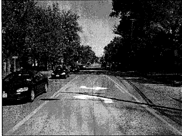
Figure 5-11 Discontinuous Sidewalks on Fuller Road
